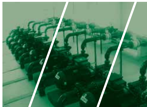
Boosting and Distribution of surface water
