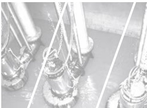
Wastewater Transport and Treatment
